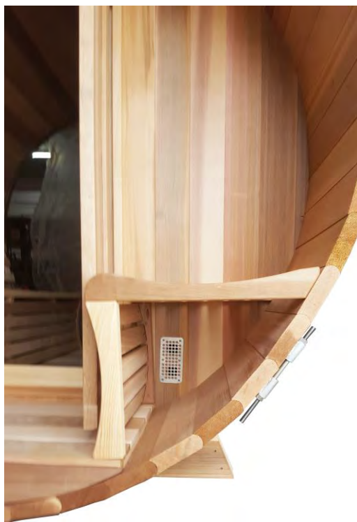
Inlet Vent on front wall
