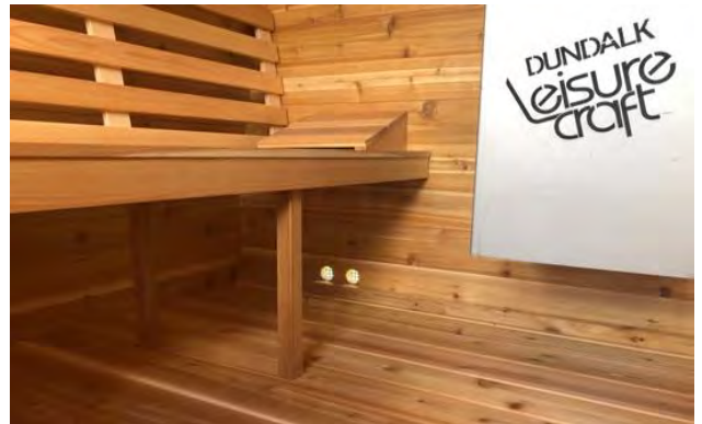
Inlet beside wood heater on Back wall
